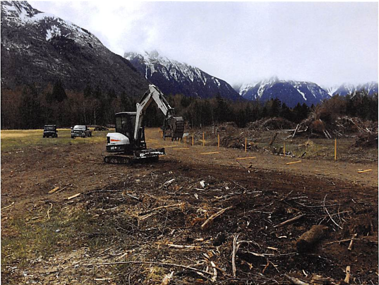
Photo: Contractor Mitch Lorimer prepares the ground for riparian planting at the west end of the airport property.
