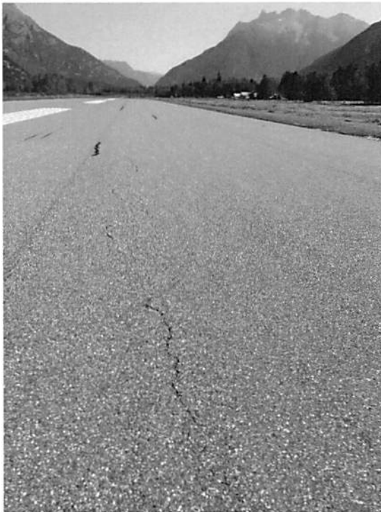
Photo 9: Low Severity un-sealed Longitudinal Cracking
