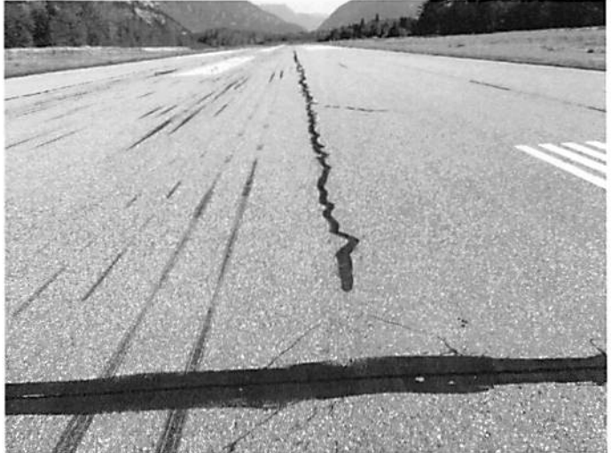
Photo 8: Transverse and Longitudinal Cracking (Sealed)
