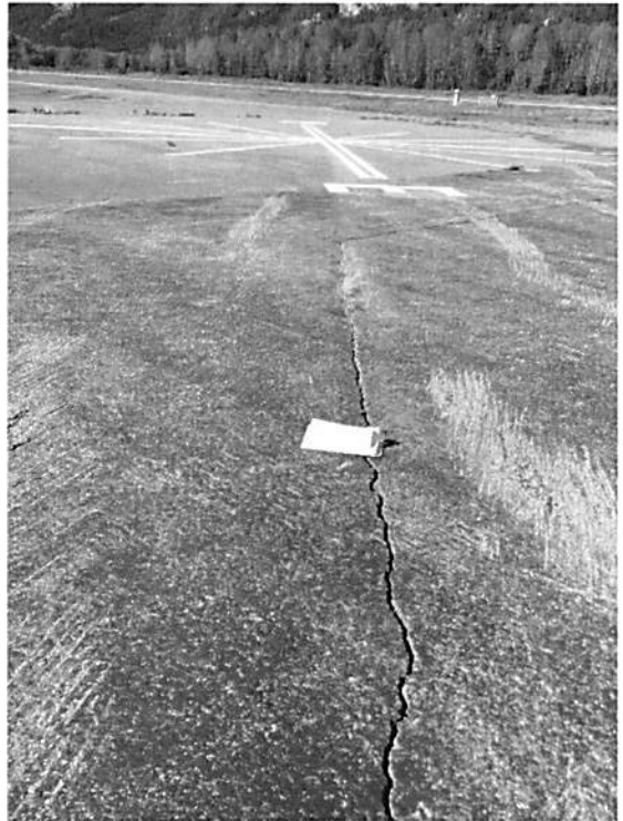
Photo 27: Moderate Crack on Apron I. Requires Sealant
