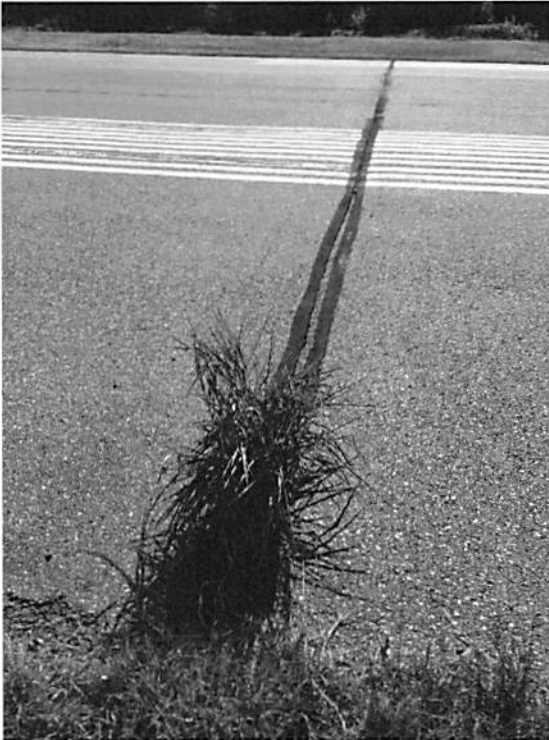
Photo 7: Vegetation Growth to be Removed
