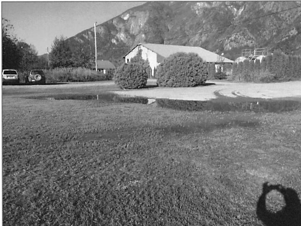
Photo 46: Settlement and Ponding in Gravel Parking Area
