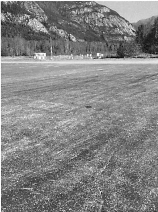
Photo 18: Low Severity Cracking on Apron I
