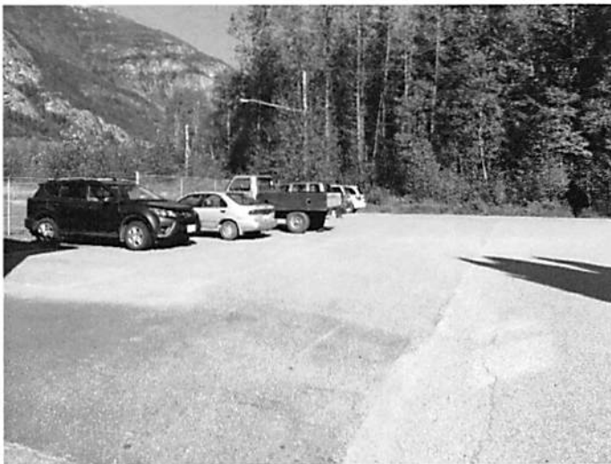
Photo 44: Cracking and rough Surface in Terminal Parking Area
