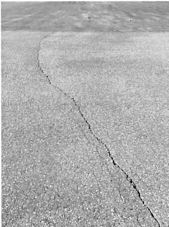
Photo 16: Low Severity Crack Apron I
