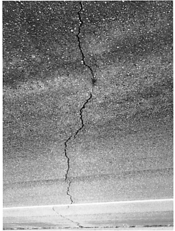
Photo 33: Transverse Crack on Taxiway B
