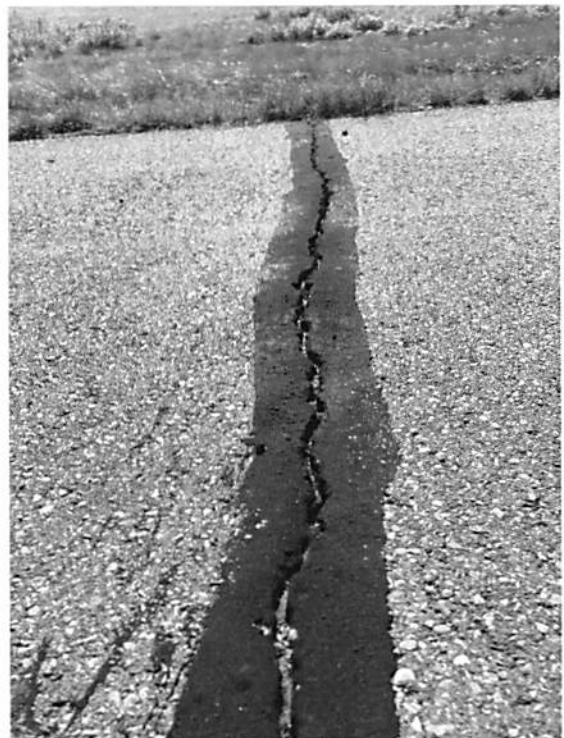
Photo 10: Transverse Crack Requiring Re-Sealing
