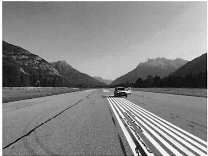
Photo 5: Low Severity Longitudinal Cracking
