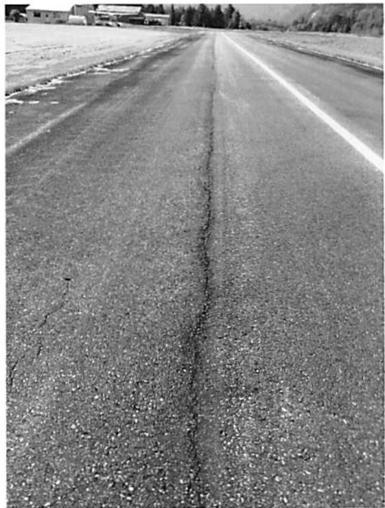
Photo 32: Unsealed Crack on Taxiway B
