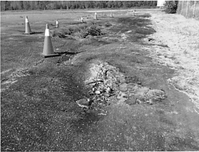
Photo 36: Major Settlement at Apron Tie-Down Area
