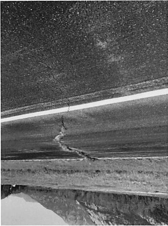
Photo 34: Crack Requiring Vegetation Removal and Sealant on Taxiway B
