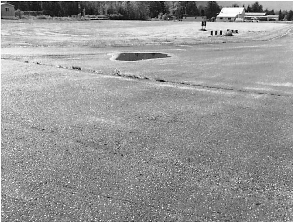
Photo 30: Ponding and Settlement on Taxiway B
