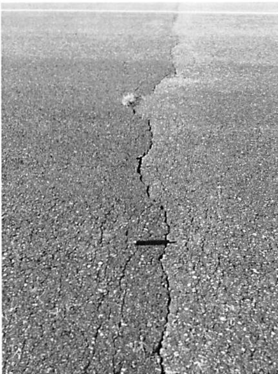
Photo 21: Transverse Crack on Taxiway A
