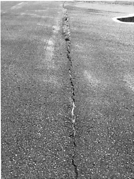
Photo 31: Unfilled Crack on Taxiway B
