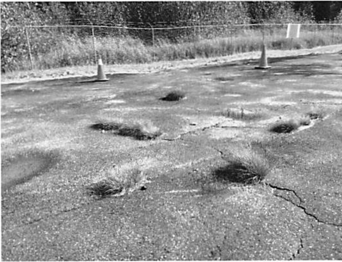
Photo 37: Major Settlement at Apron Tie-Down Area
