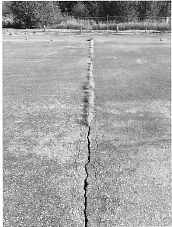
Photo 19: Vegetation Removal and Crack Seal Required on Apron I
